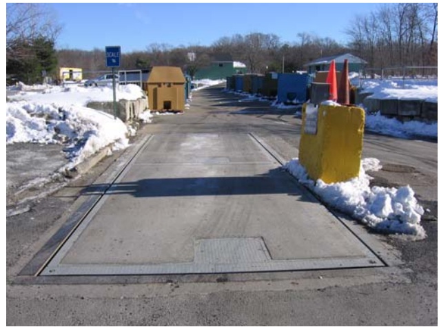
RTS Scale Replacement
