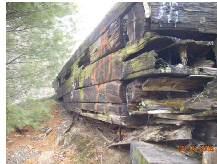
Figure 54: Deteriorated Northwest Abutment
