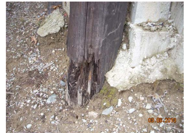
Figure 55: Deteriorated Timber Pile and Soil Erosion at Abutment
