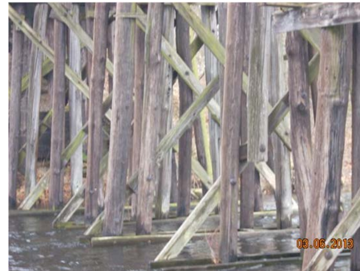
Figure 52: Missing Timber Piles
