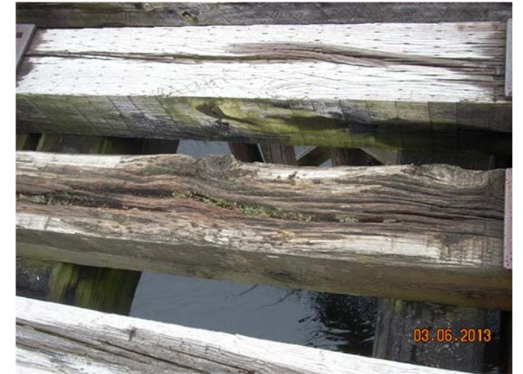
Figure 53: Deteriorated Timber Ties
