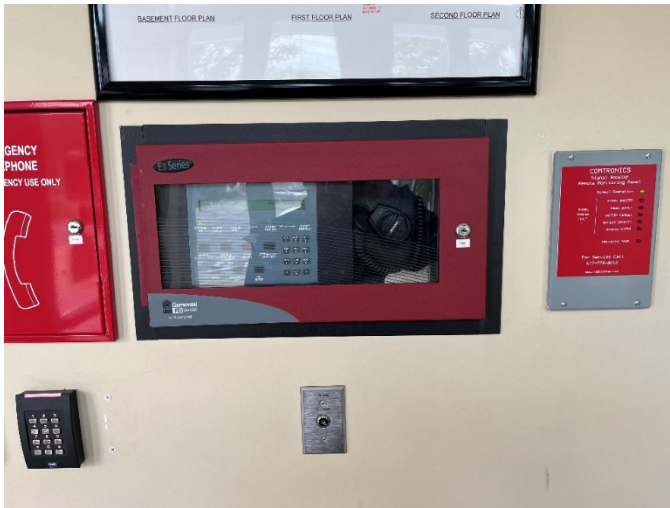
Existing Fire Alarm Control Panel
