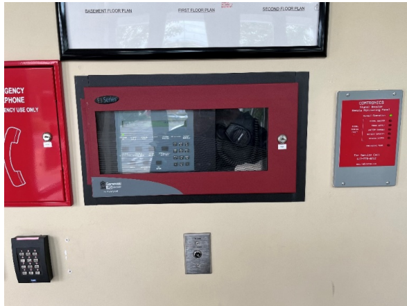
Existing Fire Alarm Control Panel
