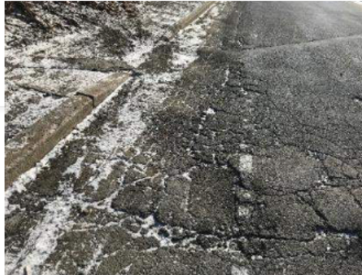
Site paving is in extremely poor condition
