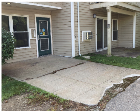
Site paving is in poor condition
