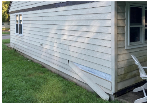
Deteriorated Captain Cook Siding
