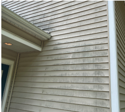
Water damage at facade
