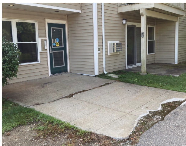
Site paving is in poor condition
