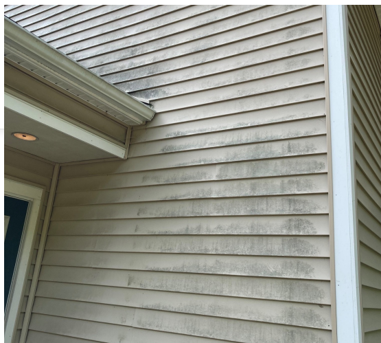
Water damage at Seabeds facade
