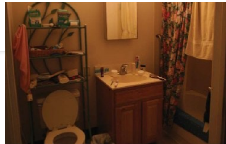
Bathrooms are worn and out of date
