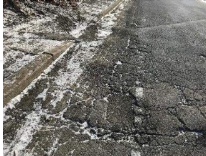
Site paving is in extremely poor condition
