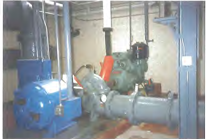
St. Mary's Street Pumping Station - Pump No. 3
