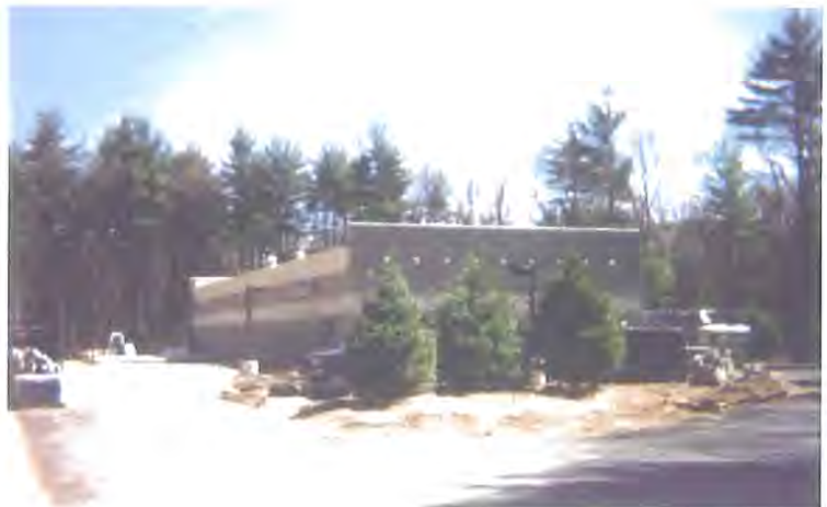
New Greensand Filtration Plant
