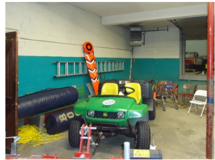
15. GAS FIRE UNIT HEATER-CART GARAGE
