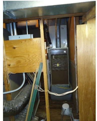
20. SECOND FLOOR – HVAC AHU
