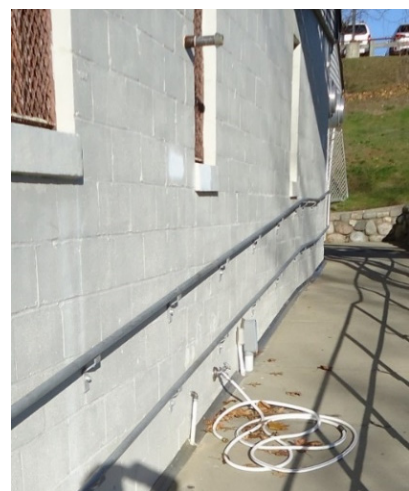
8. UNKNOWN TERMINATION AND PIPE EXITING WALL EXTENDING UNDERGROUND.
