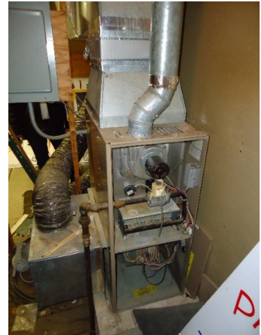
19. SECOND FLOOR – HEATING ONLY AHU.
