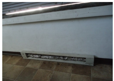
18. DAMAGED ELECTRIC BASEBOARD RADIATION AT CONCESSION AREA (KITCHEN)
