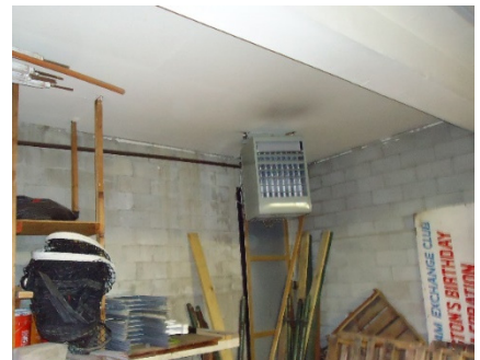
16. GAS FIRE UNIT HEATER-GARAGE1
