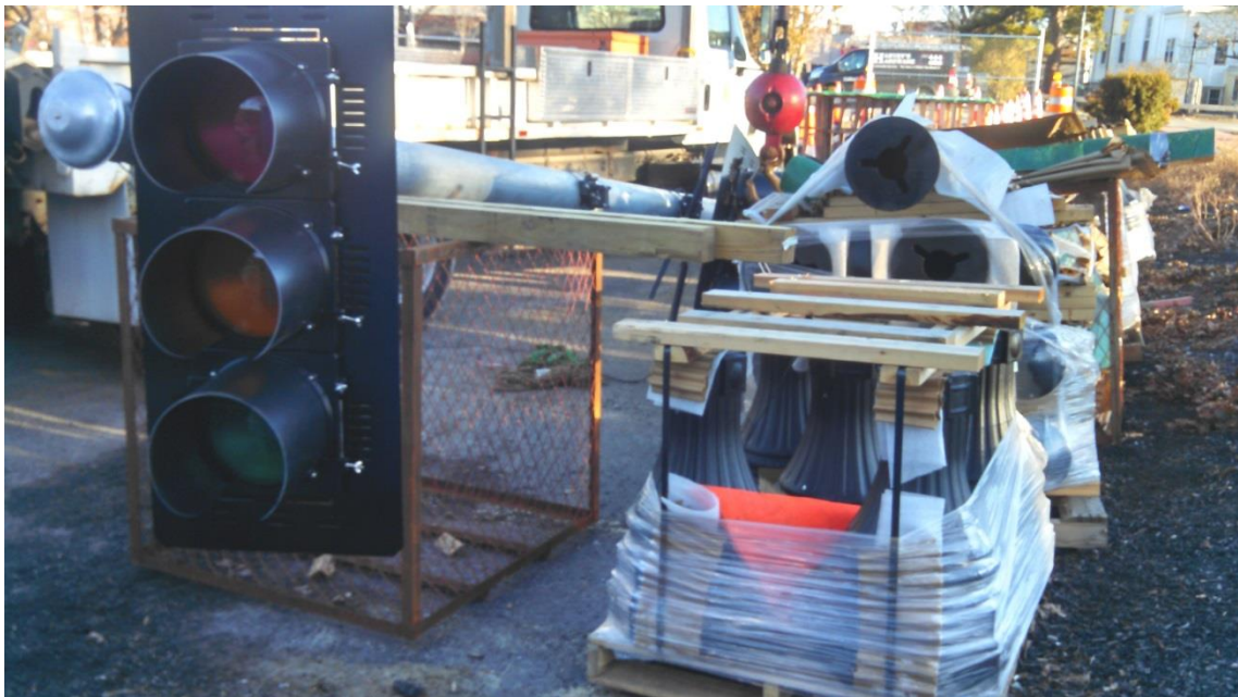
Traffic signal equipment being stored at the staging area
