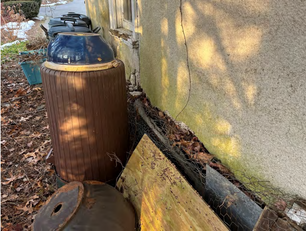
Photo 1: Crack in garage wall. Photo taken on 01/21/22
