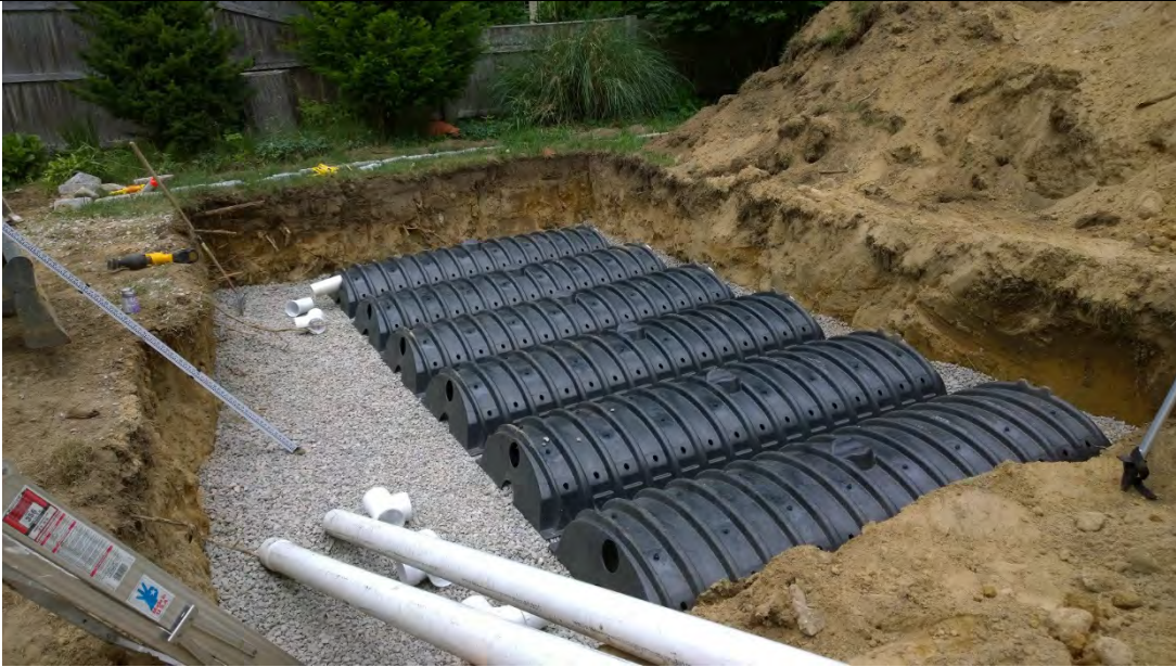
Photo 5: Subsurface infiltration system for roof runoff installed behind house. Photo taken June 2015.
