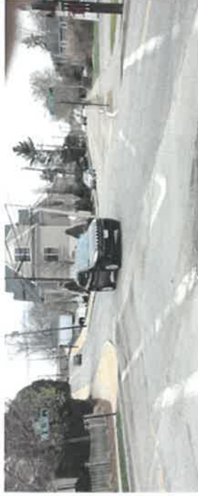
Faded pavement markings at Hunnewell/Hillside
