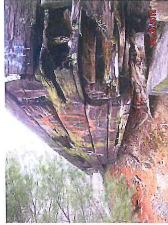
Figure 54: Deteriorated Northwest Abutment
