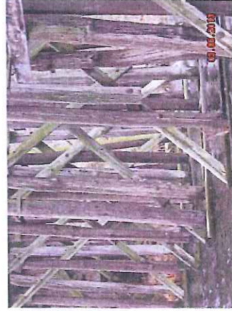
Figure 52: Missing Timber Piles
