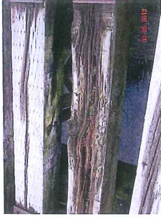
Figure 53: Deteriorated Timber Ties
